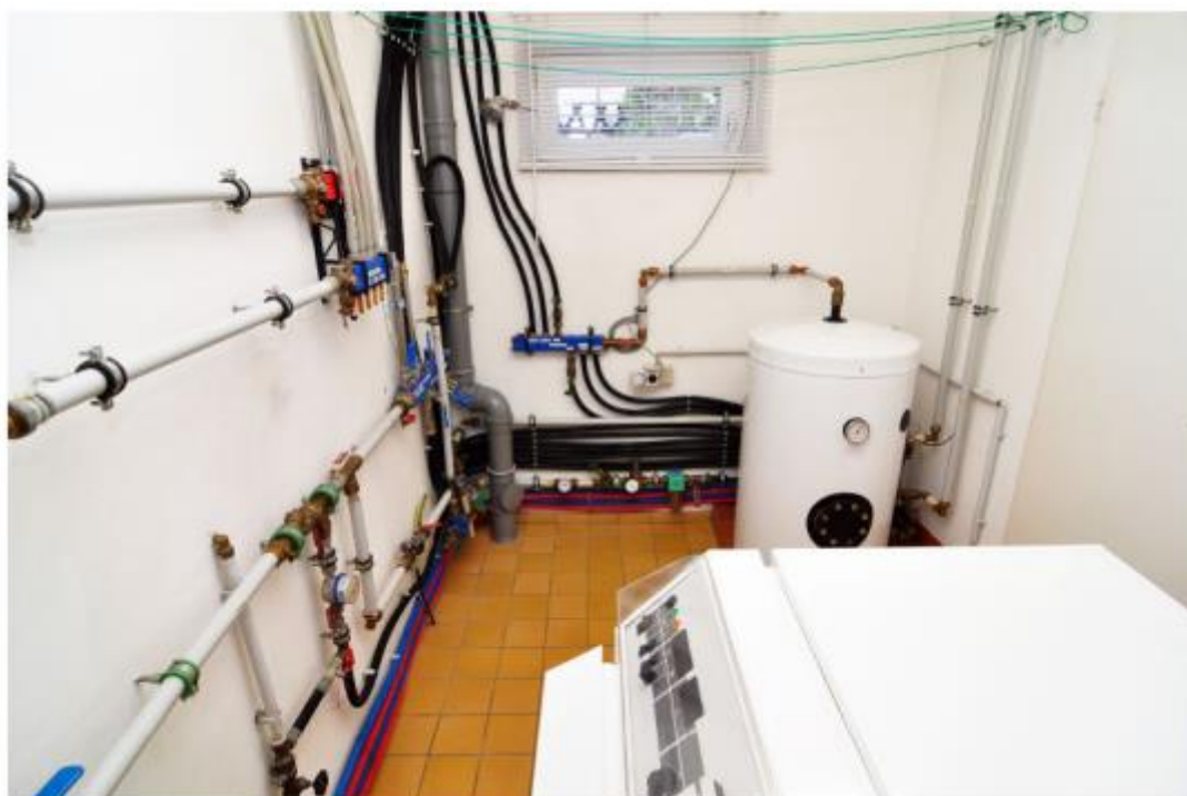
Photo 10 - Heating System - Sample Street XX, ZIP Sample City
